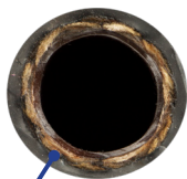
Reinforcing Cord Deterioration
